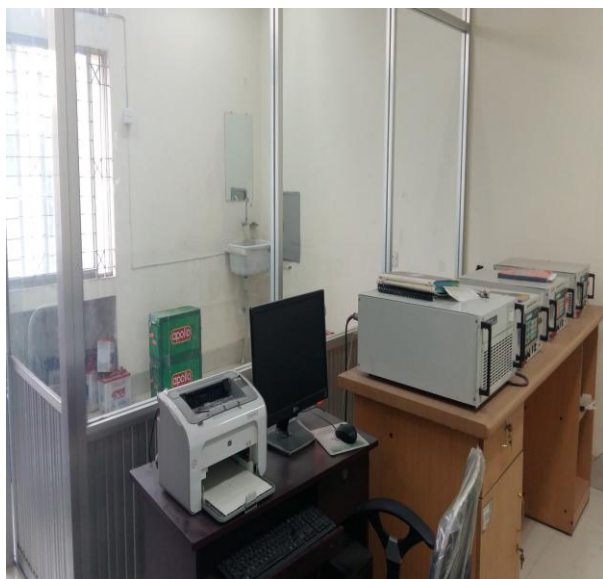
LAS Battery Testing Equipment ( another view )
