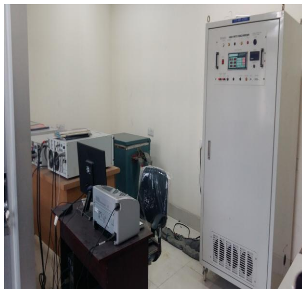
LAS Battery Testing Equipment
