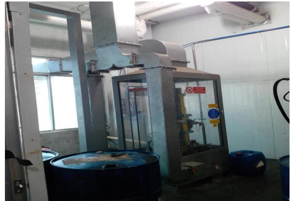
Picture : Unit-2 Premixing Exhaust System
